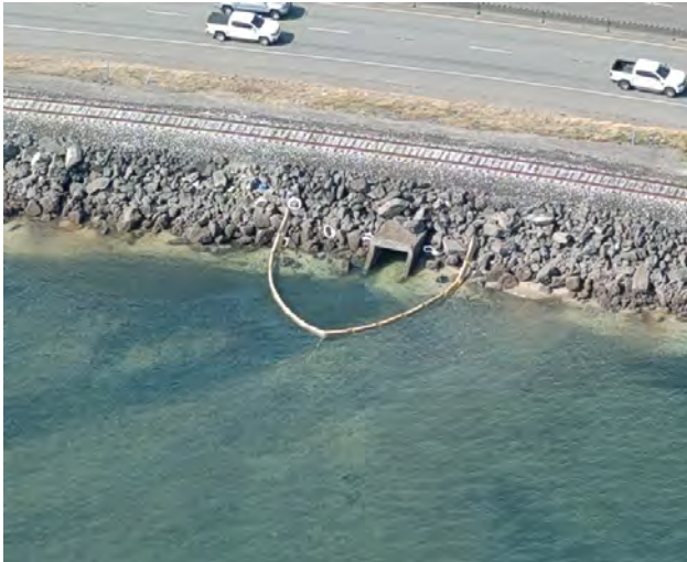
CPS-83f Photo: From above Sinclair Inlet, looking west toward outfall. Photo was taken during incident in September 2025.
