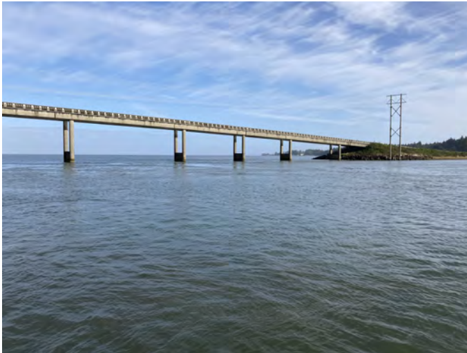
GH-9 Photo: From Elk River, looking northeast towards eastern end of bridge. Photo was taken in early October.
