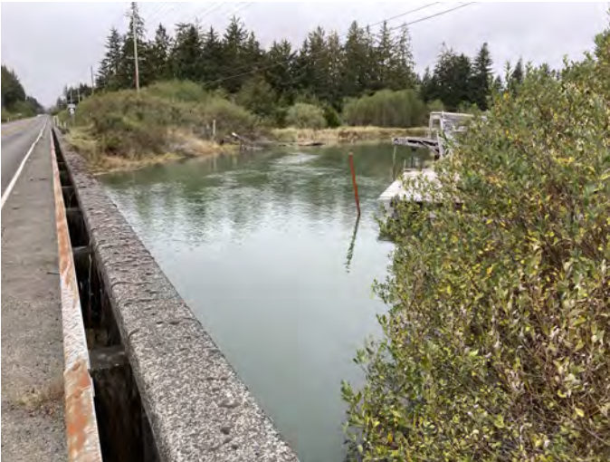
CHNC-0.1R Photo: At east end of bridge, looking north across the creek towards anchor point A. Photo was taken in early October.
