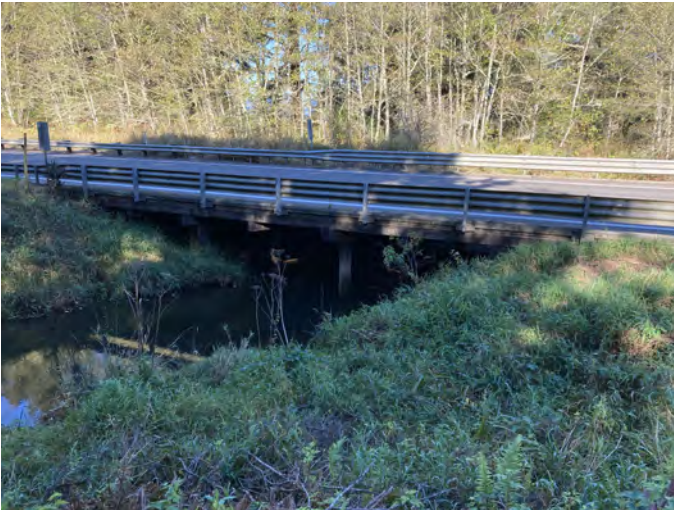
CMBC-0.1 Photo: From right bank of creek, looking northwest/downstream towards bridge. Photo was taken in early October.
