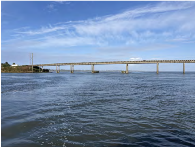
GH-10 Photo: From Elk River, looking northwest towards central end of bridge. Photo was taken in early October.
