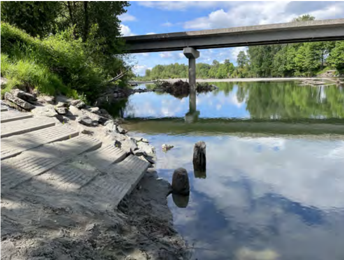
SA-STLGR-17.7 Photo: Haller Park boat launch ramp in Arlington on the Stillaguamish River. Ramp has a steep drop off and is not suitable for trailered boats.
