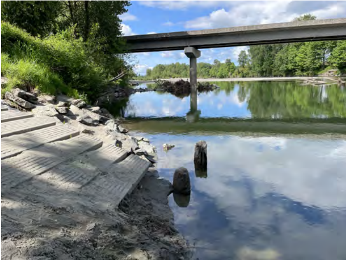
SA-STLGR-17.7 Photo: Haller Park boat launch ramp in Arlington on the Stillaguamish River. Ramp has a steep drop off and is not suitable for trailered boats.
