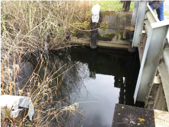
SAMR-27.0 Photo: From river right (Point A), facing E towards river left at strategy location, downstream of bridge. Taken at high spring water.
