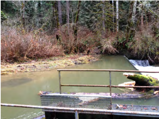
FRIC-1.7-N Photo: From Friday Creek right, looking N at fish ladder and spillway at water intake diversion dam.
