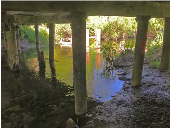
FRIC-9.6 Photo: From creek left under road bridge, facing N upstream towards creek right at strategy location. Taken at average spring water.
