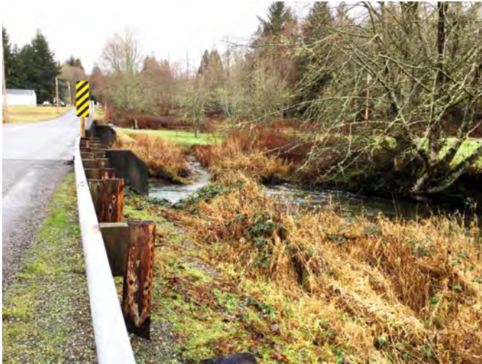
FRIC-2.4 Photo: From creek right, facing N towards strategy location on downstream side of road bridge. Taken at low winter water.
