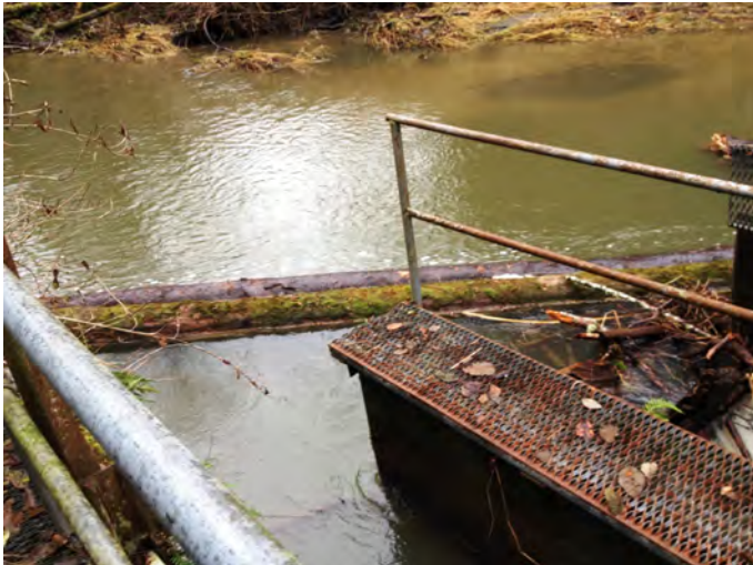
FRIC-1.7 Photo: From creek right on top of water intake, facing NW upstream towards log boom and top of fish ladder. Taken at low winter water.
