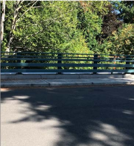
COALC-0.5 Photo: Facing NNW and Lake Washington downstream on the S side of the bridge over creek.
