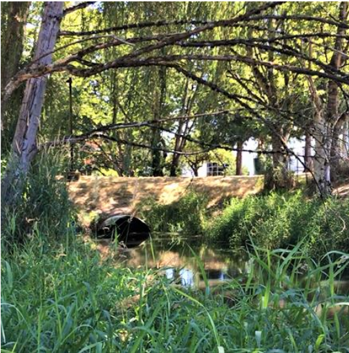
NCTRB-0.3 Photo: Facing downstream at culvert from the SW side of North Creek at Sports Field 1.
