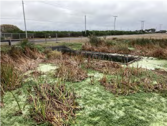
GH-1 Photo: From dock on canal, looking southeast towards culvert. Photo was taken in early October.
