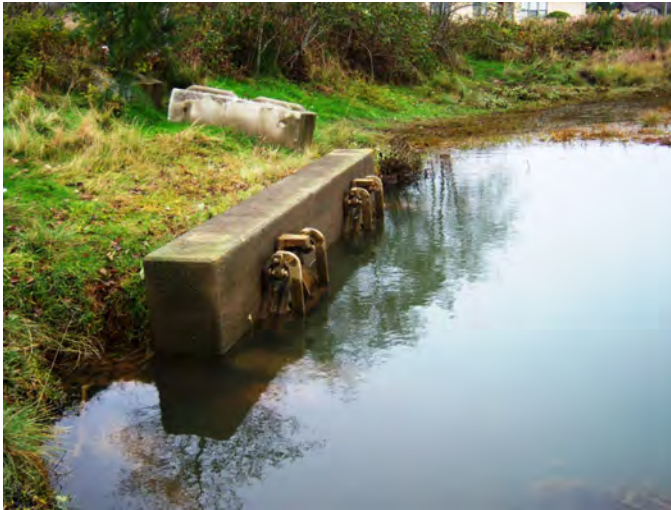
GH-02-N Photo: Looking west towards outer tidal flood gate located. The gate is normally closed at high tide.
