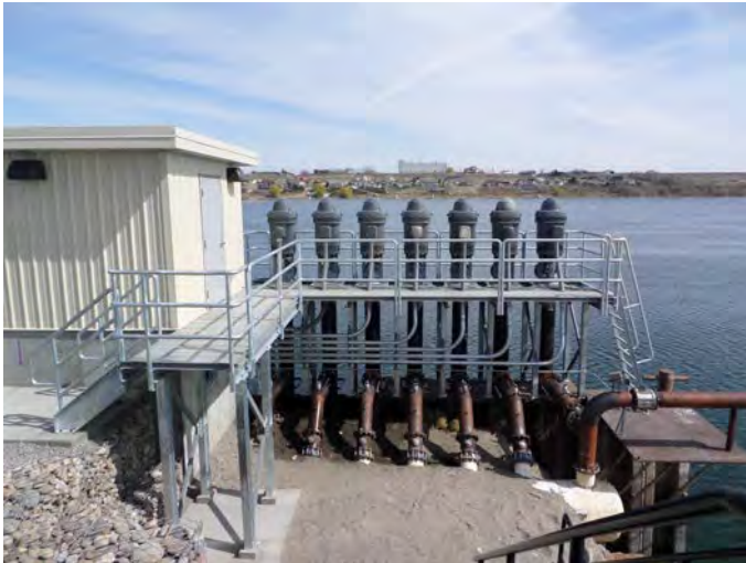
M-343.0-N Photo: The N. Richland irrigation water intake facility
