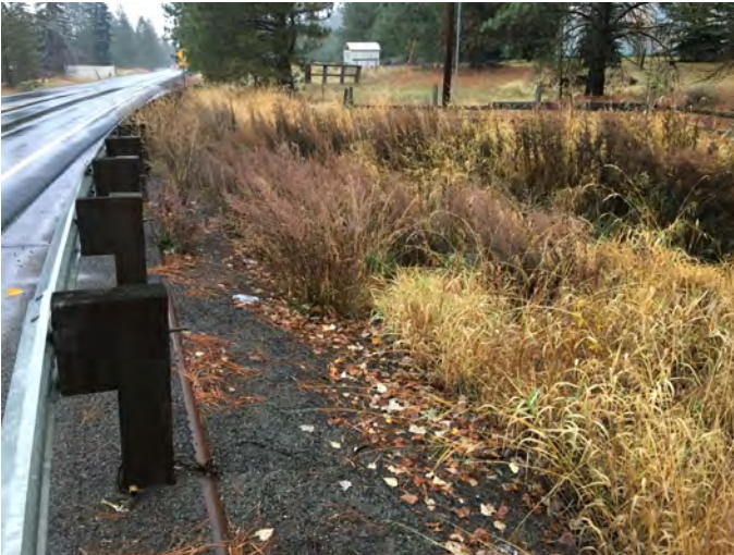
MHC-3.2 Photo: From eastern side of S Cheney-Spokane Road on Marshall Creek left, looking north towards location of culvert block.
