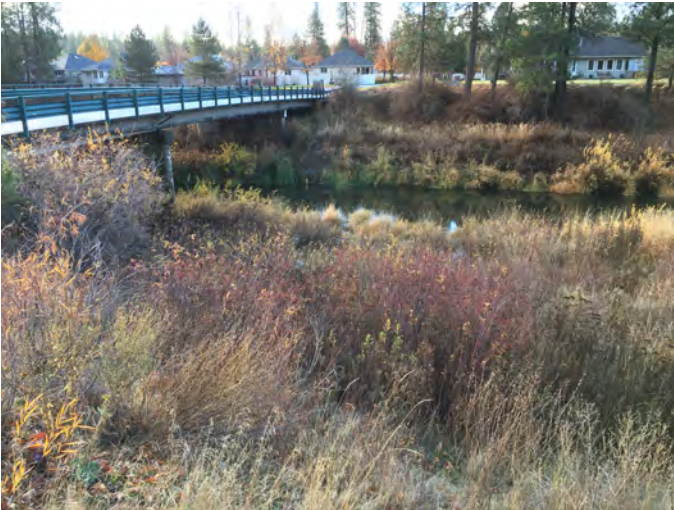
HMC-6.2R Photo: From park road on Hangman Creek right, looking upstream towards bridge and anchor point A.
