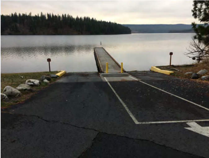
SA-SPR-38.1R Photo: From top of boat ramps on Spokane River right, looking at boat dock with left bank in the background.
