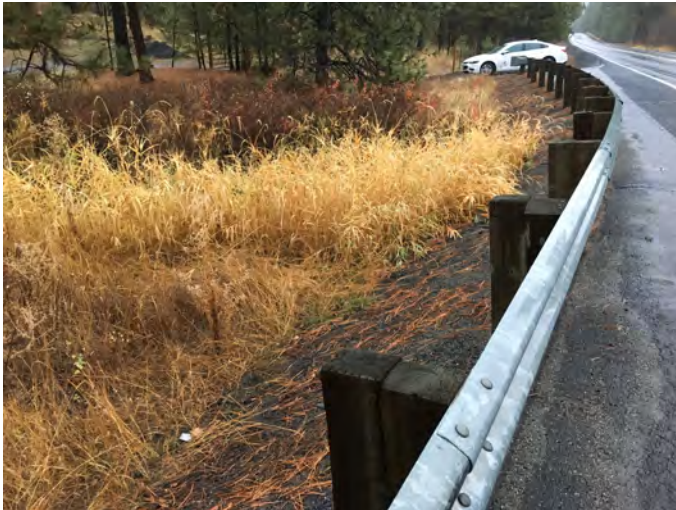
MHC-4.0 Photo: From western side of S Cheney-Spokane Road on Marshall Creek right, looking south towards location of culvert block.
