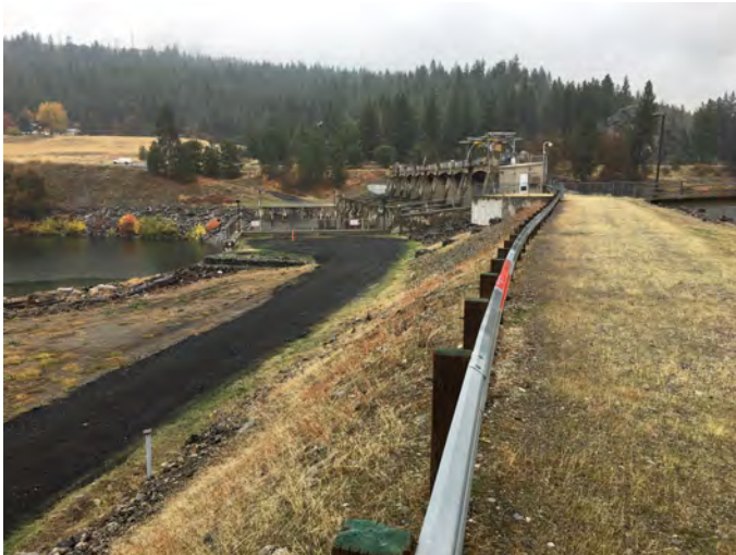
SPR-80.0-N Photo: From boat ramp in the middle of the Spokane River, looking at the dam with right bank in the background.
