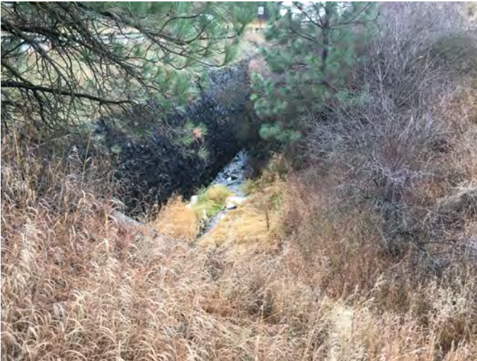
MHC-0.5 Photo: From road shoulder on Marshall Creek left, looking upstream towards ditch in which creek flows.
