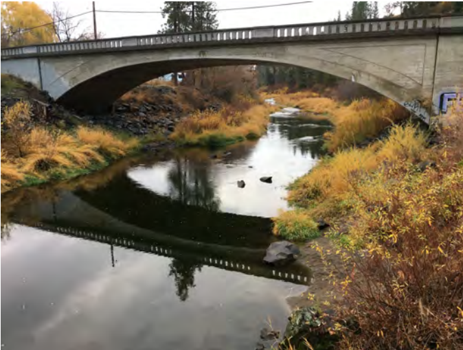
HMC-1.5R Photo: From northern/downstream side of Marne Bridge on Hangman Creek left, looking upstream toward anchor point A.
