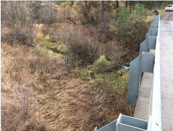
DC-9.7 Photo: From western end of bridge on Deep Creek right, looking across creek towards left bank.
