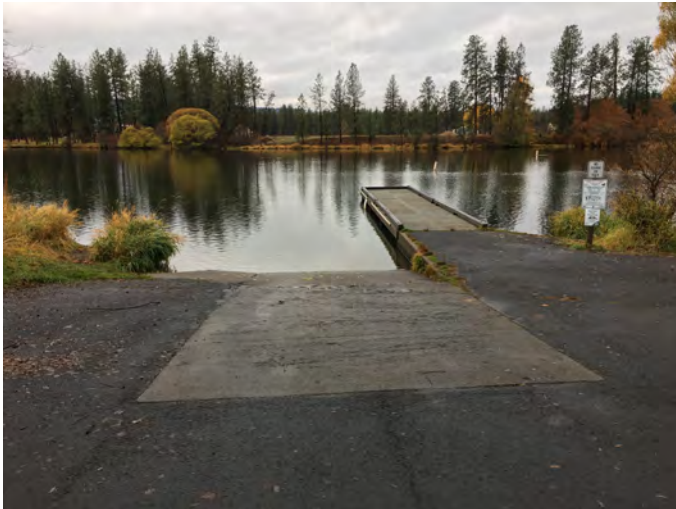
SA-SPR-56.7R Photo: From top of boat ramp on Spokane River right, looking at boat dock with left bank in the background.
